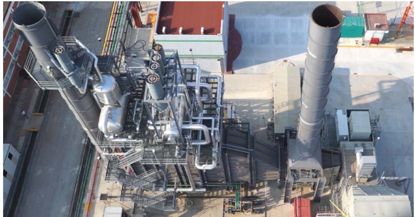
SGT-750 combined heat and power plant in Altamira, Mexico
