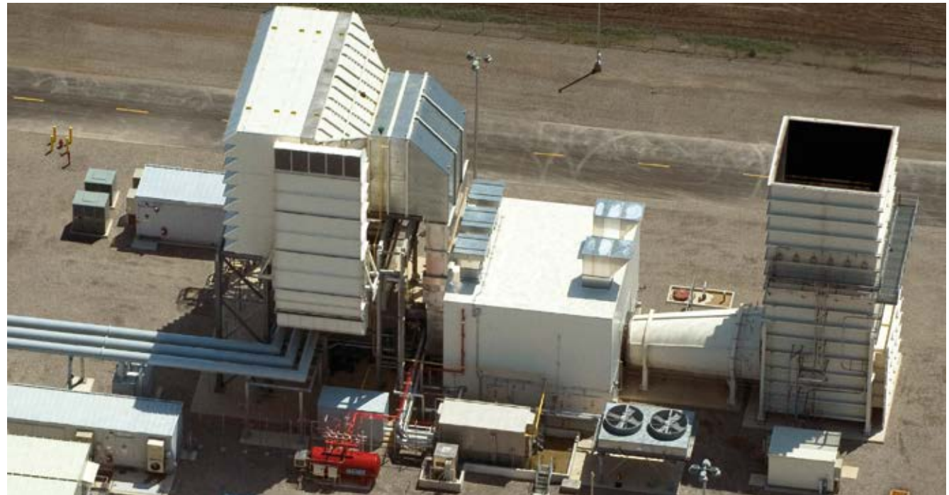
Charles D. Lamb Energy Center, Oklahoma, USA
