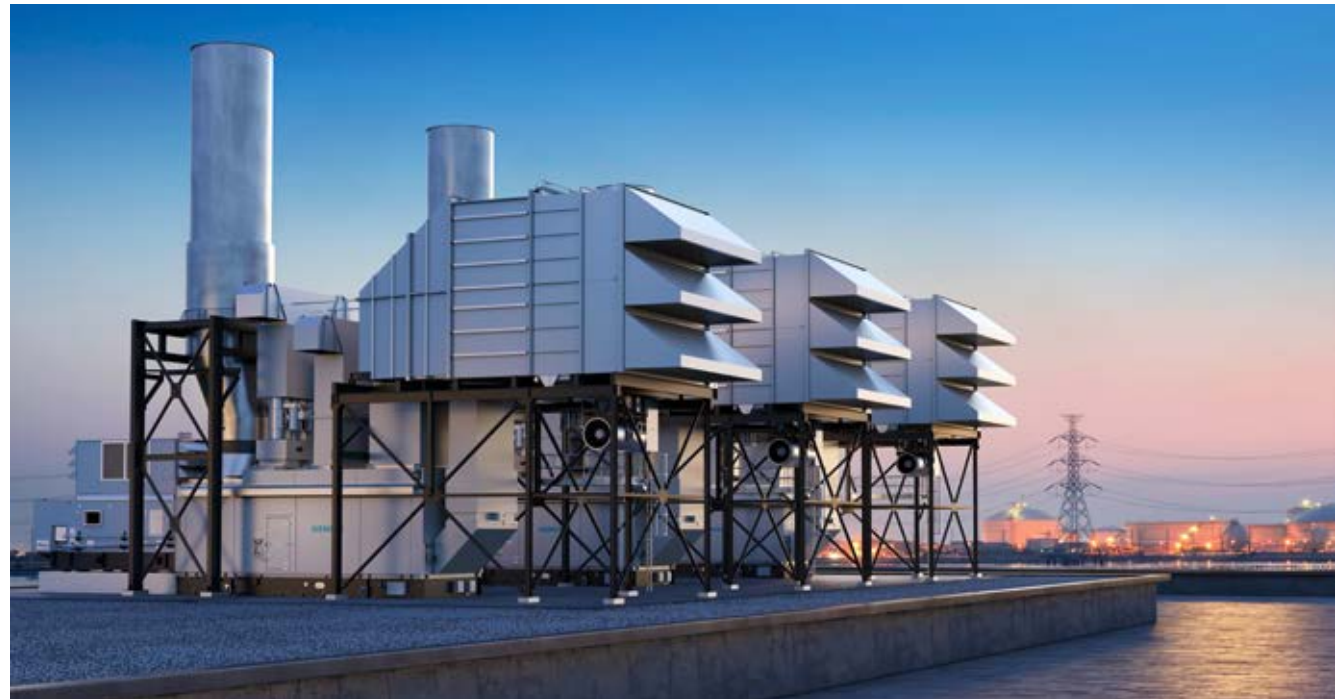
Three SGT-A65 units for power generation
