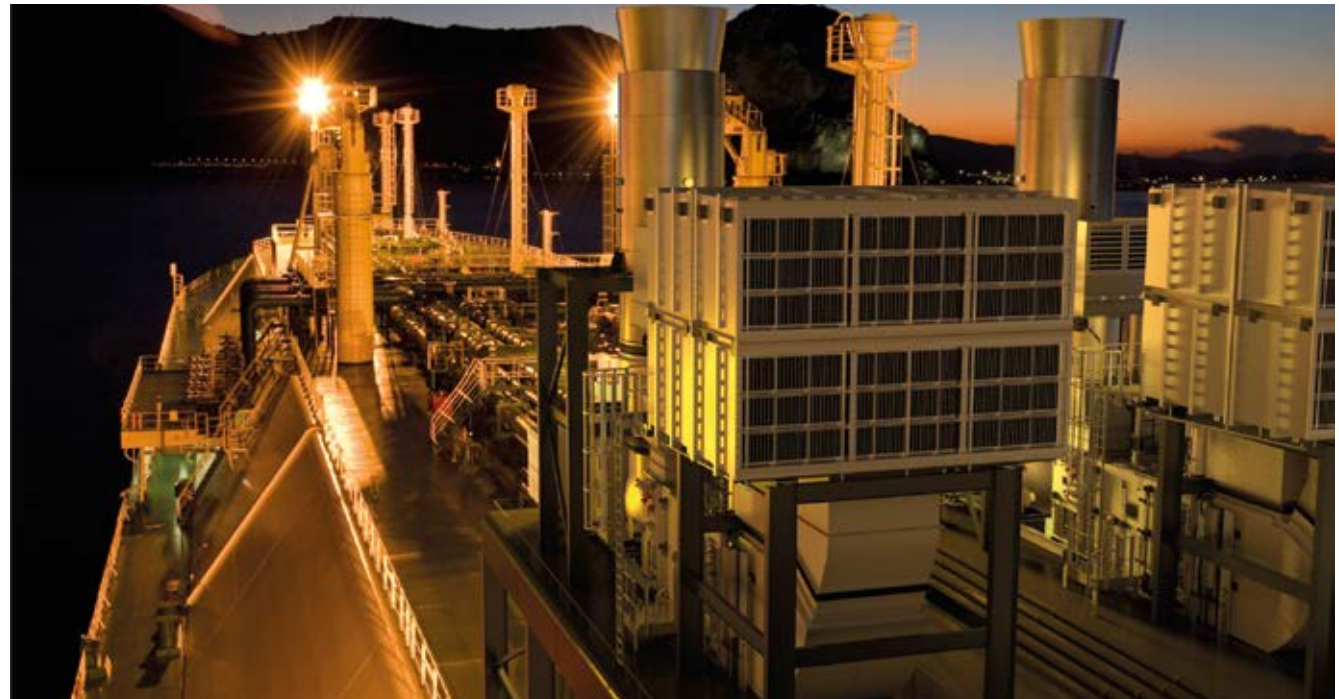
Two SGT-A35 (Industrial RB211-GT30) packages on an FPSO vessel
