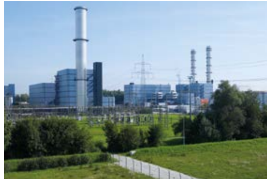
High operational flexibility due to world-class fast cold start and hot restart capability
