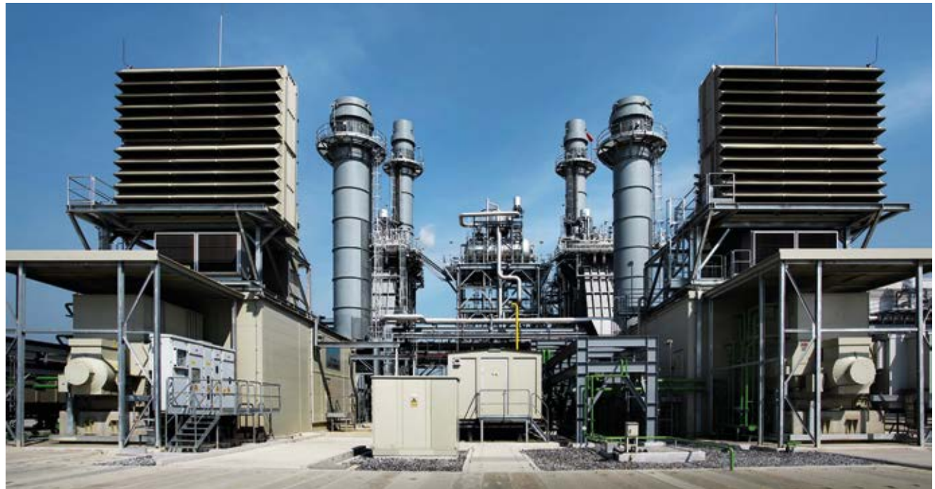
SGT-800 packages at the Amata B.Grimm Power Plant, Amata Nakorn, Chonburi, Thailand
