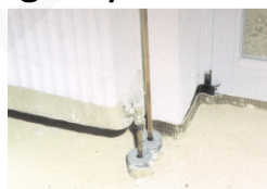
Pipe insulation in heated area (no unwanted floor heating)
